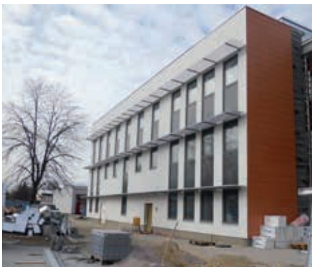
The construction of the new building of the FFPW USB and the FA USB in Na Sádkách in České Budějovice. The facilities will be servicing for education and research and development.
