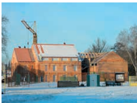
The object of the International Environmental Educational, Advisory and Information Center of Water Protection Vodňany before and during reconstruction.
