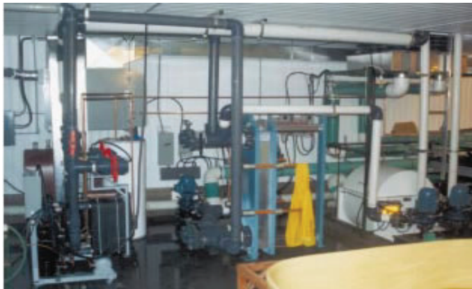
Water heating system at Alléghanys Inc.
